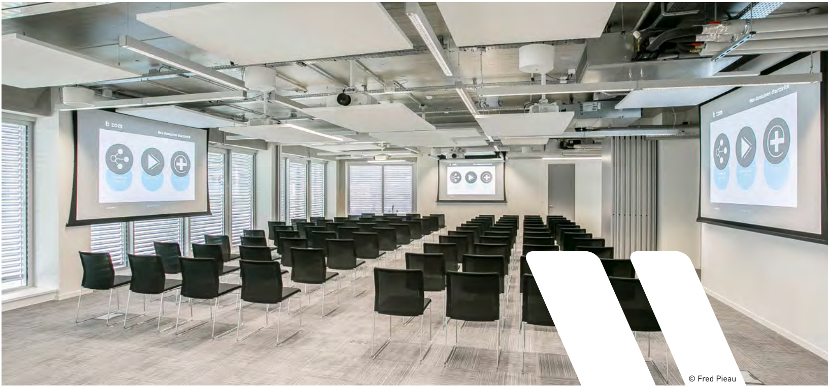
Product: Tensioned Elpro Concept Installer: Videlio Rennes Location: b<>com l'Espace Conférences (Rennes, France)
